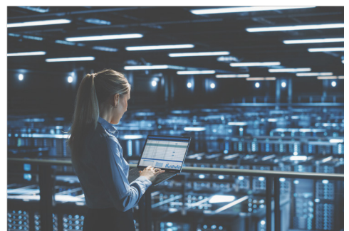
Micro Data Center & Server Room
